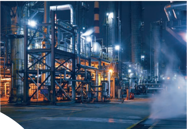
Factory-independent power supply, lower electricity bills
